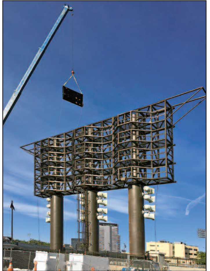
A crane lifted jumbo screen components onto the larger frame as part of the installation process. Photos by Justin Purdy
